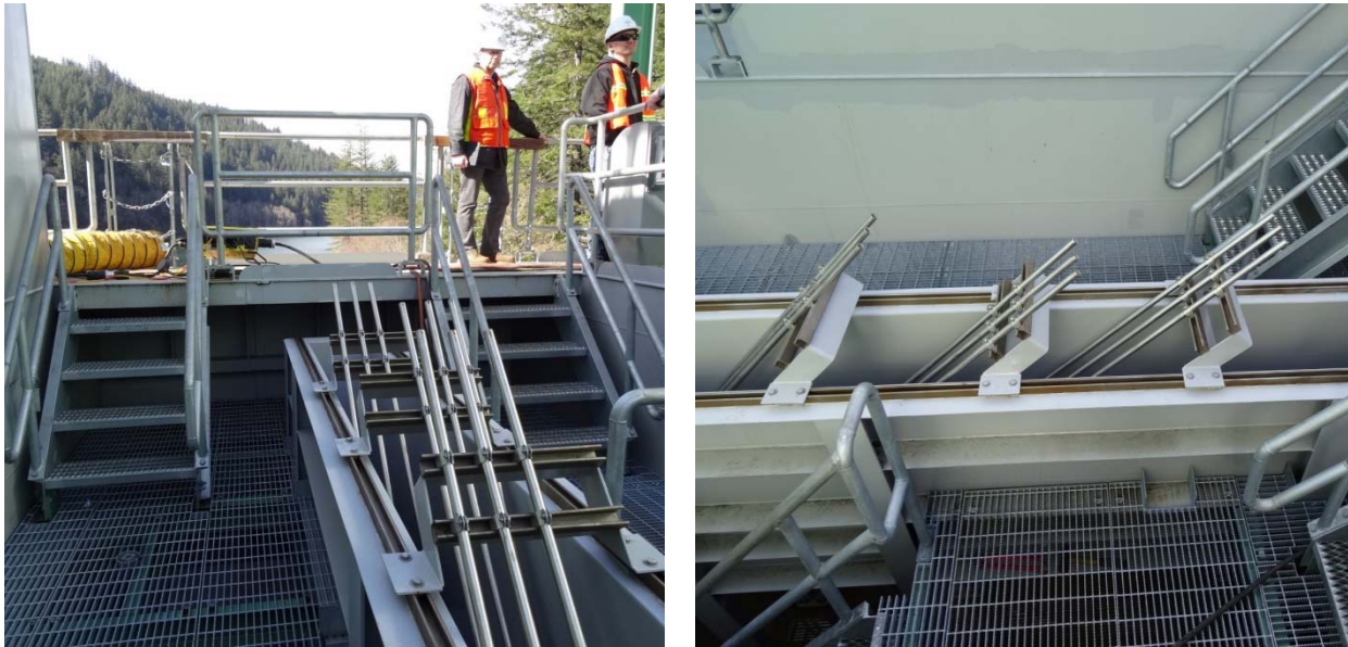
Figure 4-10 - Photos of the Debris Rack in the North Fork FSC Transport Channel
