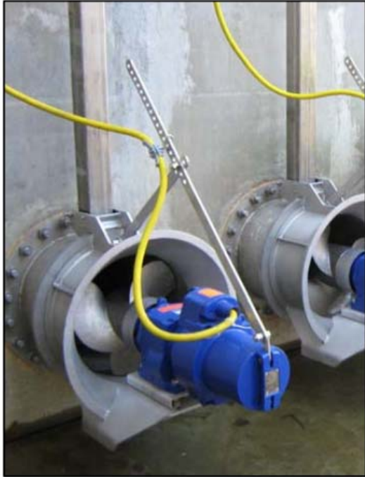
Figure 6-1 - Typical installation of Flygt mixer pumps, guard rails, & submersible power cable
