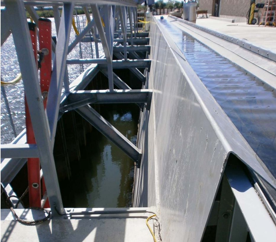
Figure6- 8. City of Stockton Intake, Automated Debris Conveyor Debris Removal System
